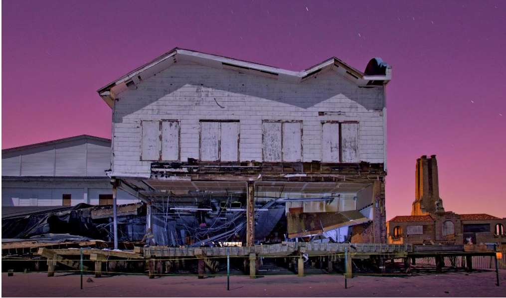
Damaged Ocean Grove boardwalk concession and the amusement steam power plant in Asbury Park. Photograph courtesy of Monmouth County resident Mike McLaughlin.
