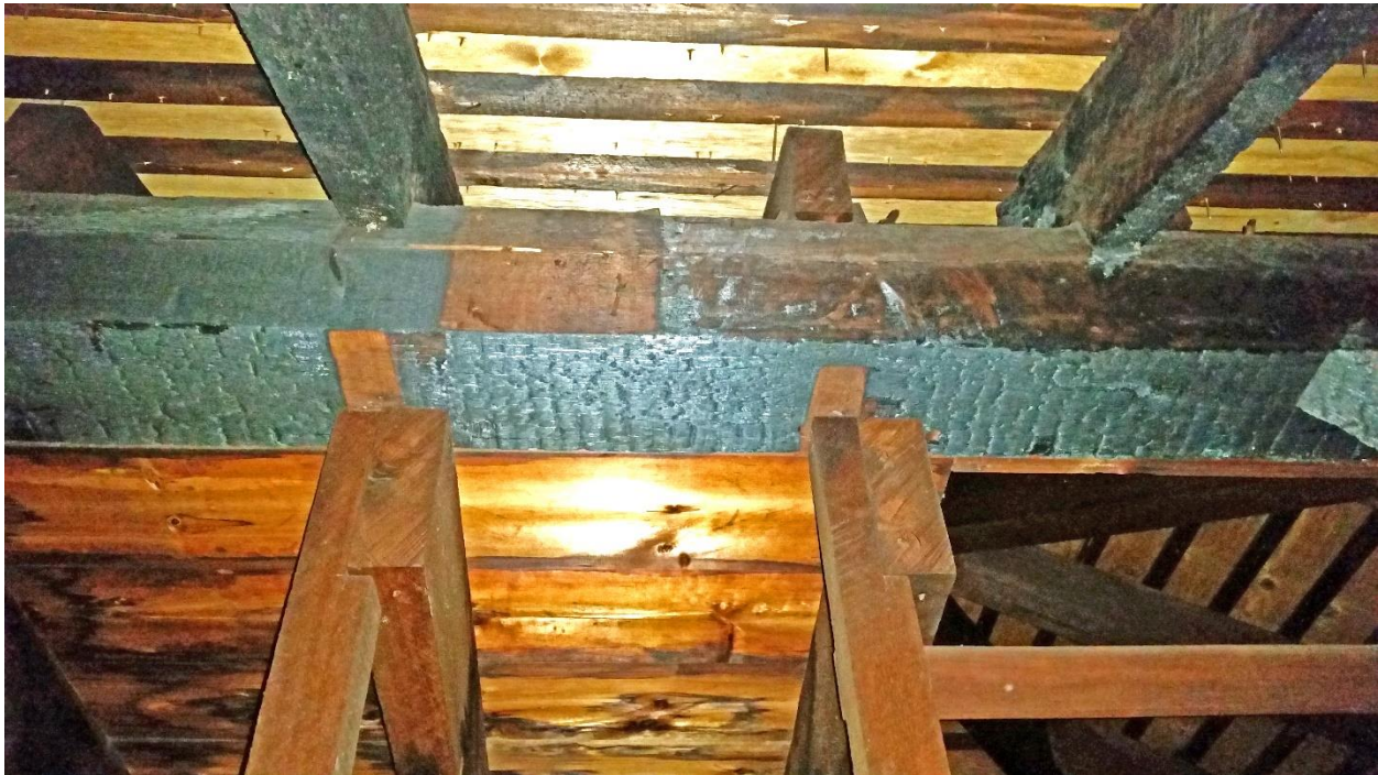
The underside of a purlin plate became charred in the 1891 roof fire at Orchard Home, as did the common rafters which are supported by it. The peak of the roof above this point required complete reframing.
