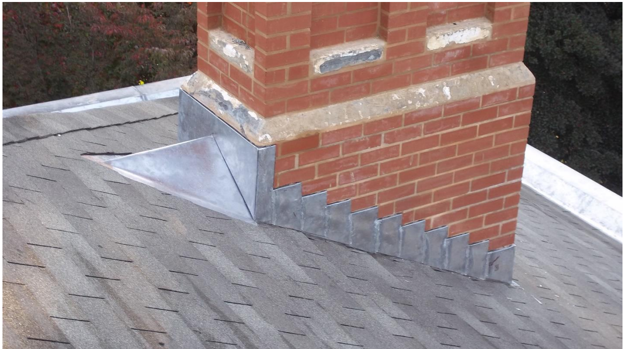
A detail showing the base of a rebuilt chimney, new flashings and gutters, and new asphalt roof shingles, 2011. MCHA image.
