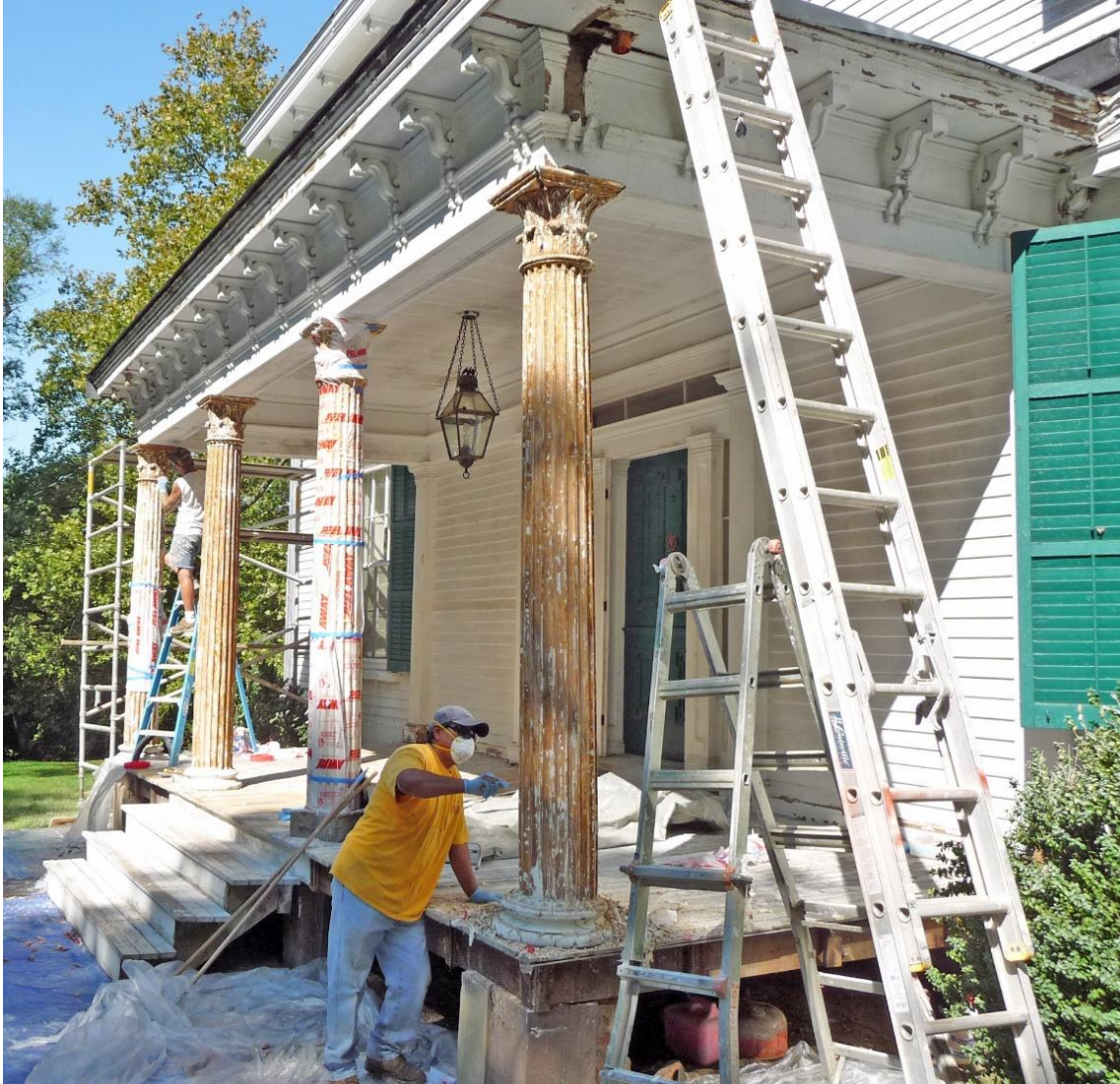
Restoration of the front porch involved removal of the thick paint accumulation from the columns and Corinthian order capitals, 2012. MCHA image.
